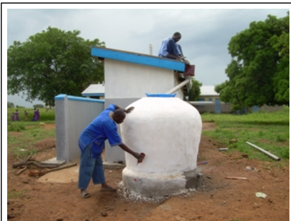
Sam and Nelson of DWU Field Crew finish the latrine and rainwater harvesting jar at Agak Primary School.
