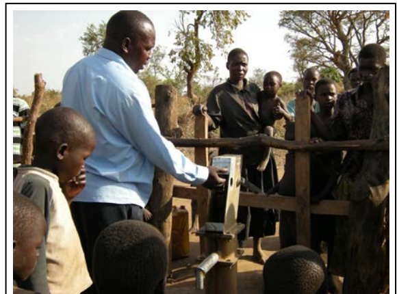
Joseph, DWU Field Crew, checks an India Mark II pump installed at Omac Abiko Village in 2010 during a previous project in Aromo Sub-County.
